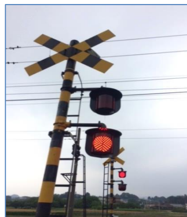
LED 踏切閃光灯
